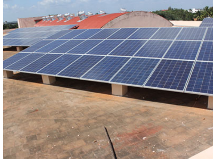
60 KW Hybrid Inverter With Battery, Tanjavur / India
