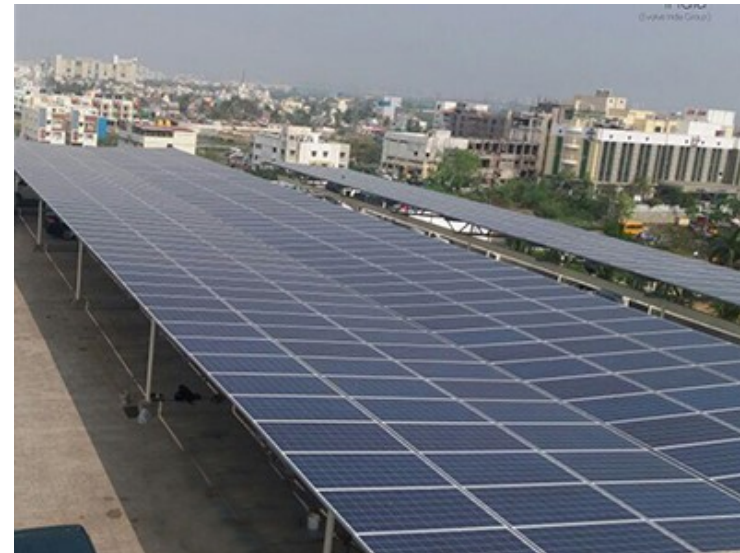
200 KW Solar Car Port, Chennai / India
