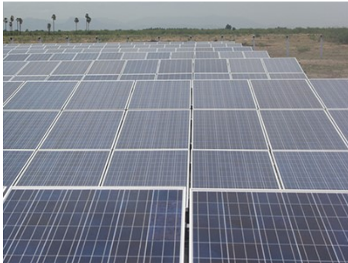
1 MW Tirunelveli / India
